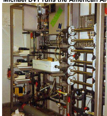
Test rack in the middle compartment
