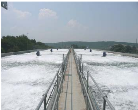
App. 1,1 MW aeration power
