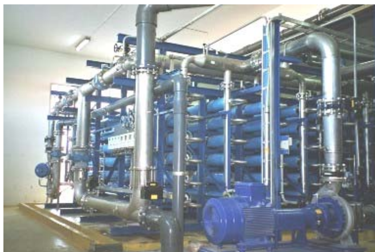
The 4 th line with interstage booster pump
