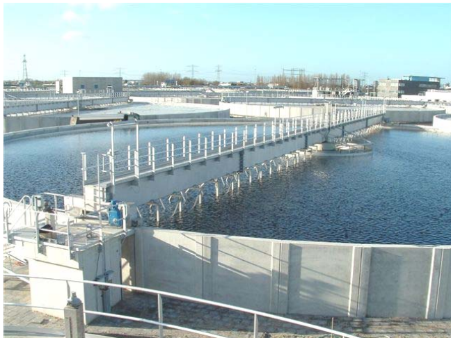
One of the 16 Secondary Clarifiers
