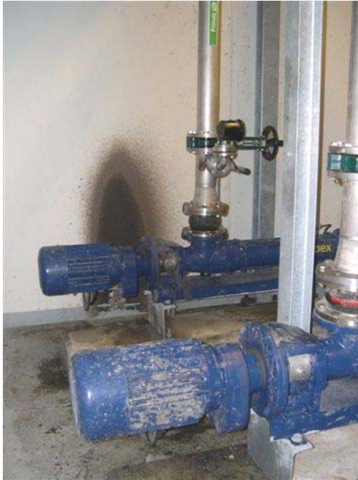
Leaking Seal (a minor upset)
